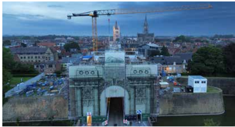
..... : The Menin Gate under restoration. : The scaffolding wrap uses an original : concept drawing by the memorial's : architect Sir Reginald Blomfield. .....
