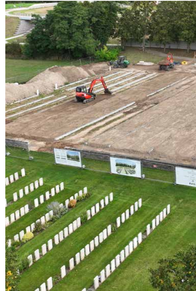
..... The beams are installed to support and align the headstones at Loos British Cemetery Extension, August 2023. .....
