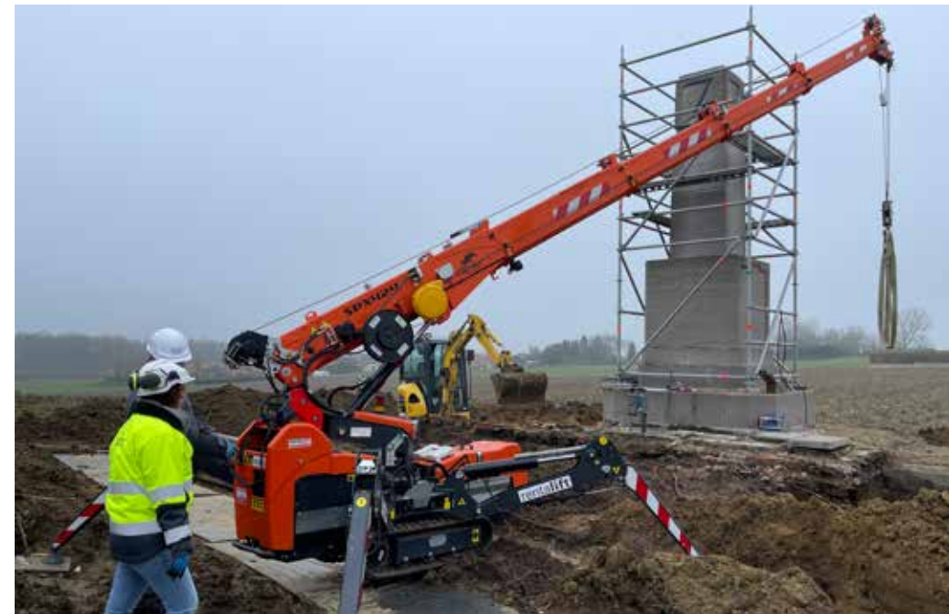
..... Restoration work underway on the 7th Division Memorial with the help of a remote control crane at Zonnebeke, Belgium, January 2023. .....
